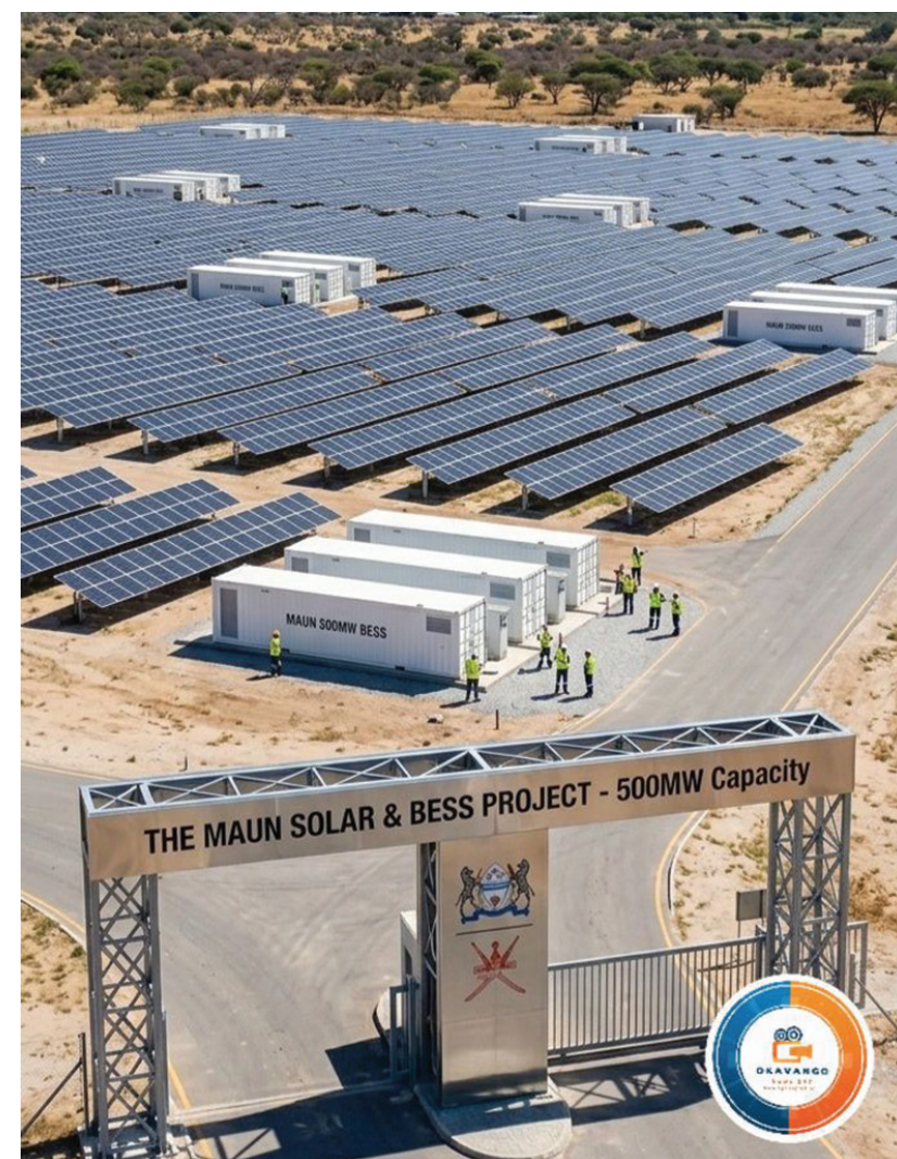
Maun 500 Mega Watt Solar Power Plant
